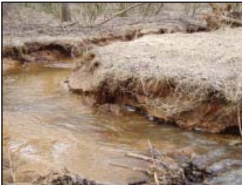
An eroding streambank along the upper section of Beaverdam Creek.
